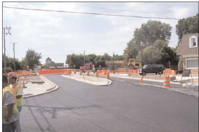
Asphalt paving of the section of Lockport Street between Main Street and James Street is completed prior to the start of the school year.
