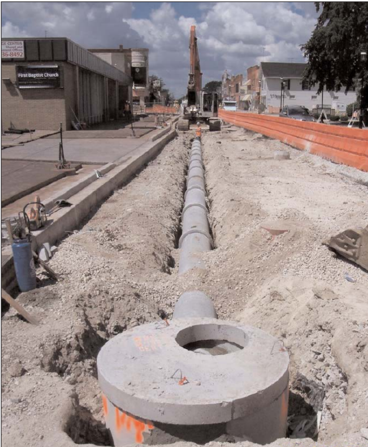
The storm sewer is extended east from Illinois Street to allow for a future connection from Route 59 as part of the upcoming IDOT improvements.
